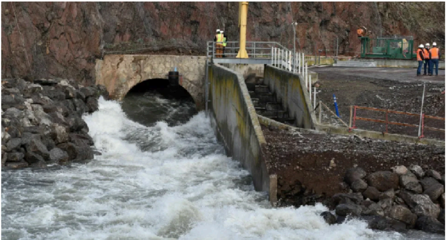
The bypass tunnel at the bottom of Iron Gate Dam in Northern California has been carefully reinforced so it can handle the load of water and sediment pouring through it. | Juliet Grable for NPR
