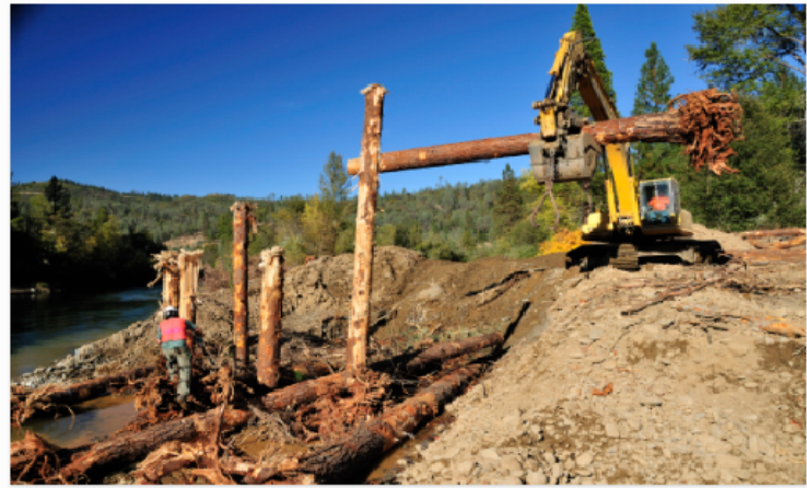
Large wood is placed at a rehabilitation site to create an engineered log jam. Photo by Kenneth DeCamp.
