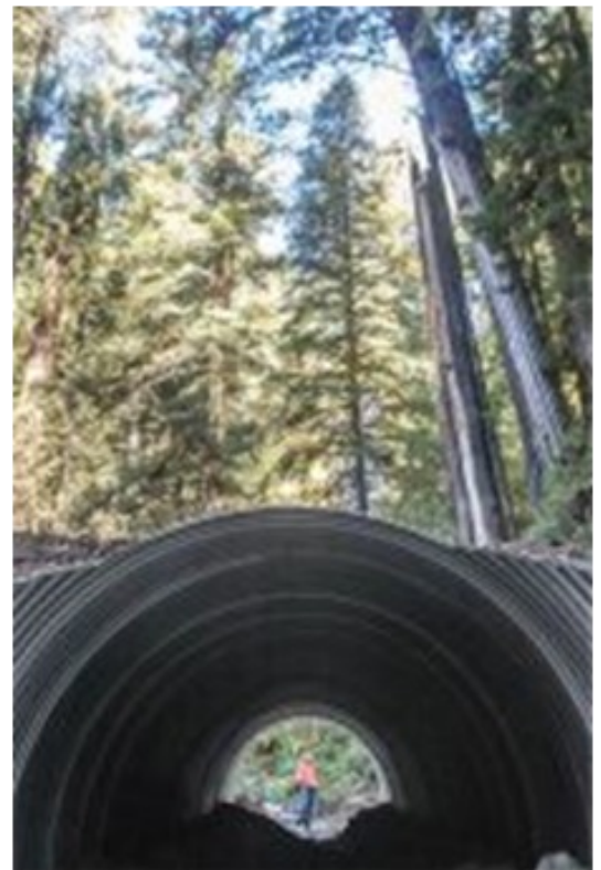
Nanette Nickerson, staff engineer for Michael Love & Associates, demonstrates culverts installed in Jedediah Smith Redwoods State Park that will open up another 2 miles of stream for fish. Del Norte Triplicate / Bryant Anderson
